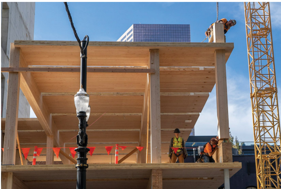
Plywood was nailed over voids between CLT panels, which along with straps, created temporary floor diaphragms so that the timber installation could proceed without the concrete topping slabs.
